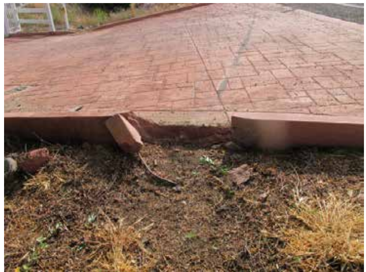
Rammed through the rebar curb!
